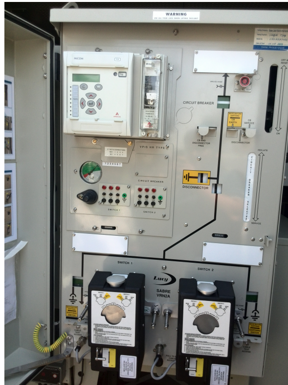
Figure 53: The TRM cabinet containing two switches to cut off supply to one side of the ring and various circuit breakers.
