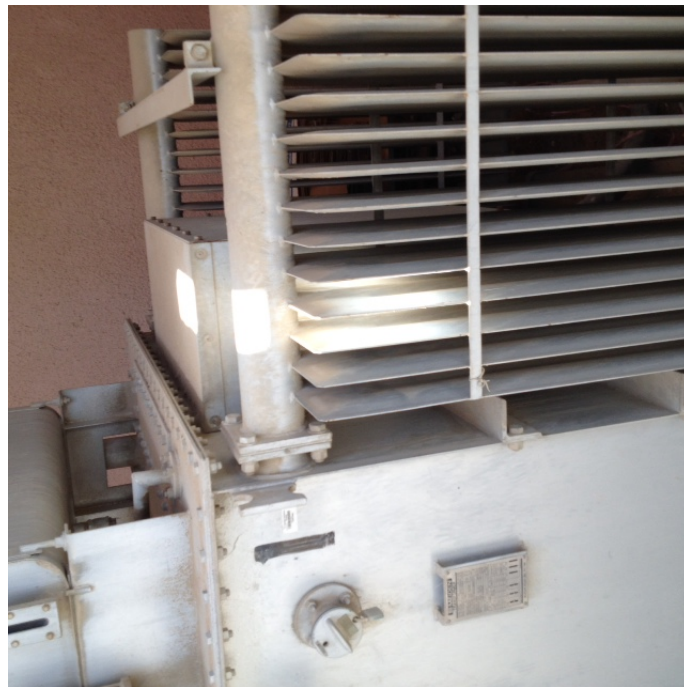
Figure 6: In the picture above, a typical step-down transformer is shown where 11kV is stepped down to 0.4kV.
