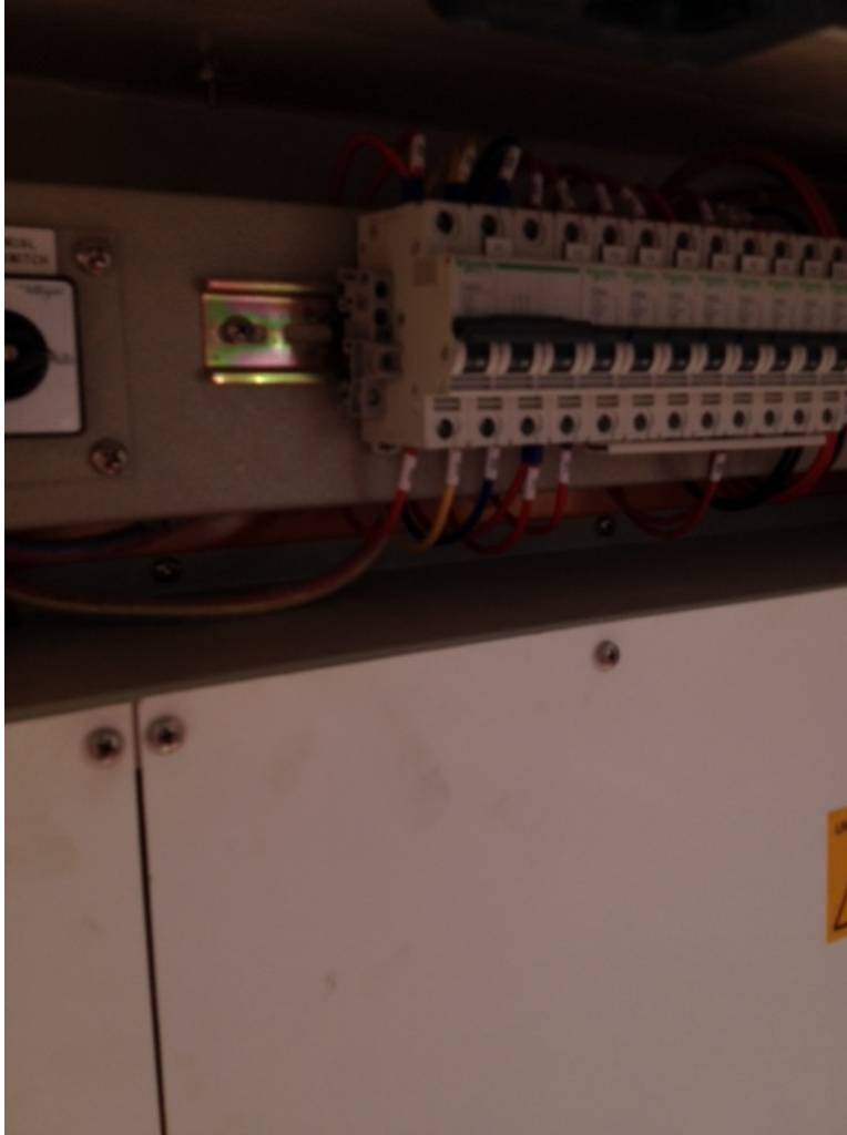
Figure 4: The figure shows the circuit breakers which are installed to protect the circuit from high current in case there is a fault.
