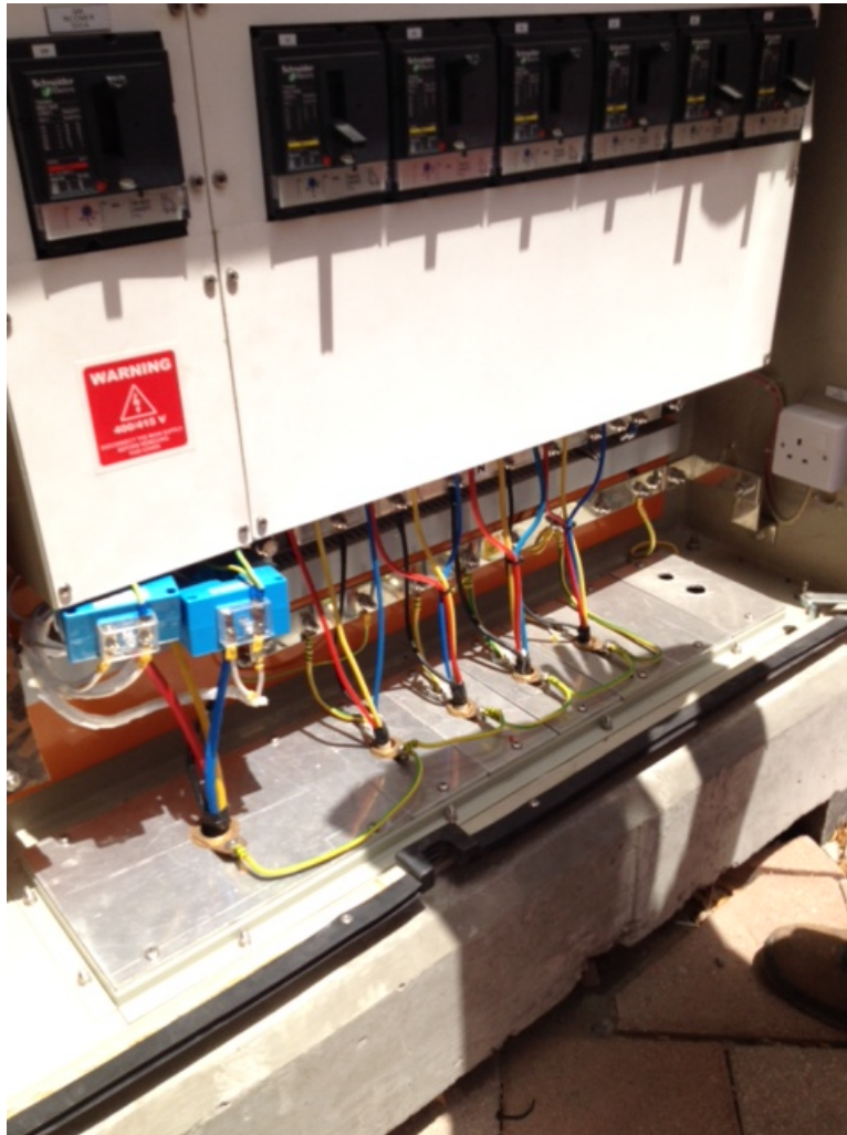
Figure 3: The figure shows the inside of the control cabinet where the switches for each sector of street lamps are installed and can be controlled either manually, by using a timer, or by photo diode. The two current transformers in blue can be clearly seen which are used for sensing the amount of current consumed by street lamps and display it on the meter.
