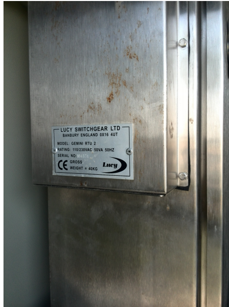
Figure 56: A separate cabinet was there for remote control using Gemini Remote Terminal Unit (RTU).
