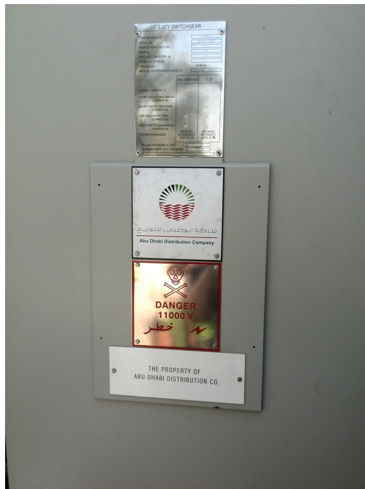
Figure 51: Outside part of the switch gear box. The Switch gear used was of Lucy brand.
