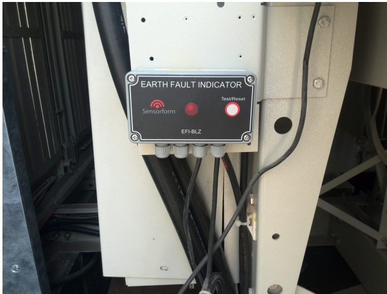
Figure 52: The Earth fault indicator attached inside the room. it works by detecting high amount of current flowing through wire by using current transformer.
