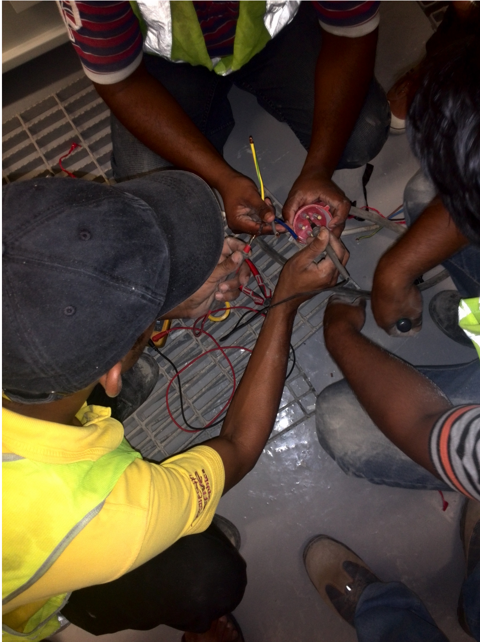
Figure 33: The voltage going in from the high voltage side of the transformer is being measured by multi-meter.
