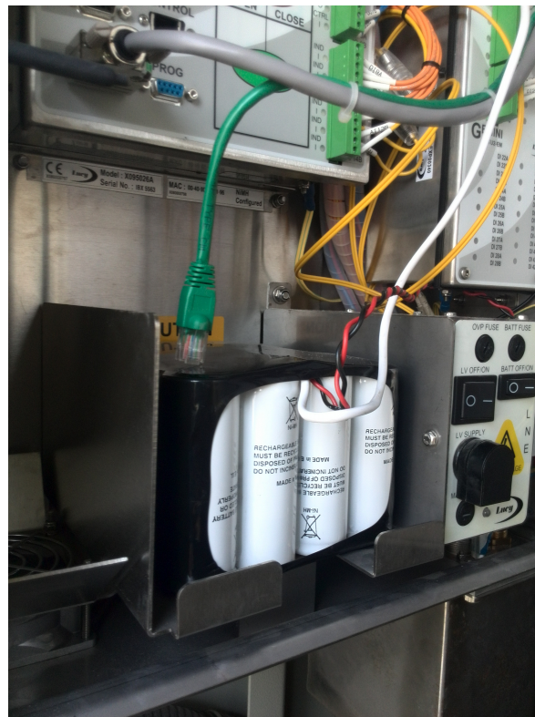
Figure 57: The RTU cabinet contains a rechargeable battery pack in case that supply is cut, the RTU is still functioning.
