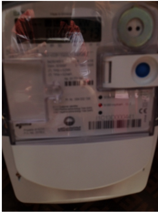
Figure 5: The figure shows the electric meter which keeps track of the power consumption of the street lamps.
