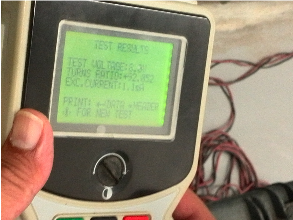
Figure 26: The turn ratio tester showing the injected voltage = 8.0V and the current = 1.1mA. The turn ratio found was = +92.052 in this particular case.
