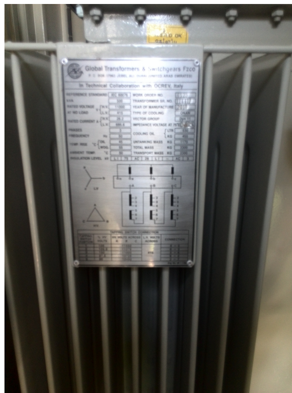
Figure 59: The TRM room contains a single transformer also for stepping down the voltage from a single point in one ring into two points in another ring.
