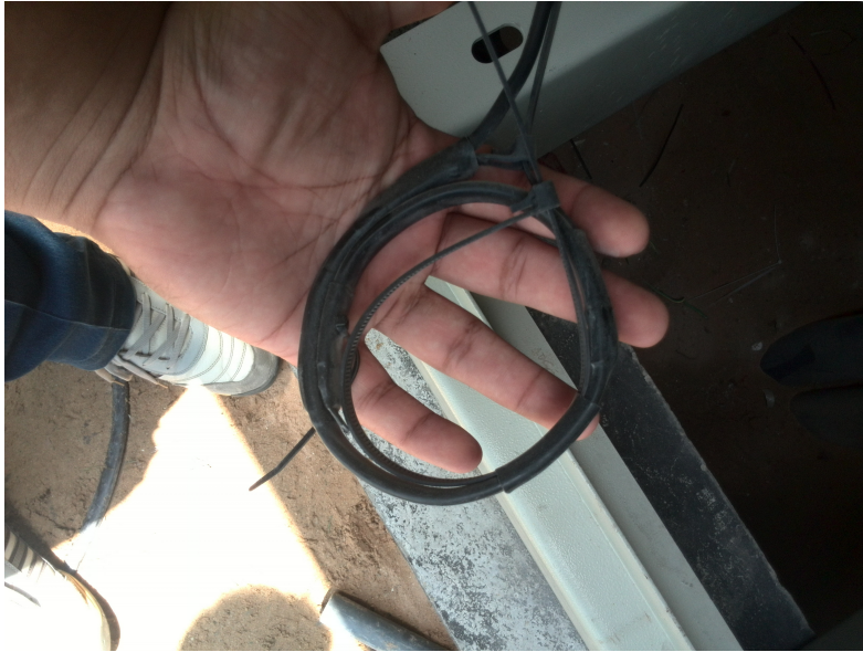
Figure 54: The Current transformer with a zip tie so that it can be tied to one of the live wires and detect the current. This with combination of a relay is used for earth fault protection when high current flow can cause damage to equipment.
